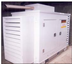
The new 40KVA generator
